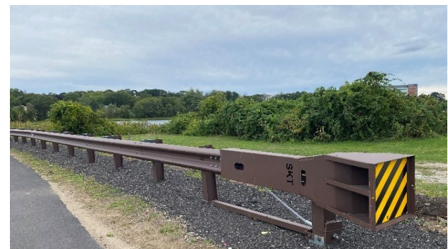
Figure 3-14 Appropriate: powder coated guardrail and end cap treatment on Veterans Memorial Parkway in East Providence, RI. Source: Pam Sherrill
