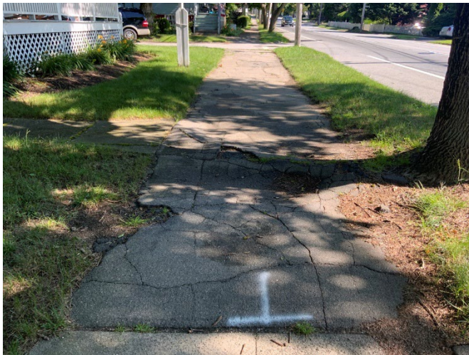
Figure 3-27. Hope Street in Bristol, RI sidewalk damage from tree roots. Source: Town of Bristol
