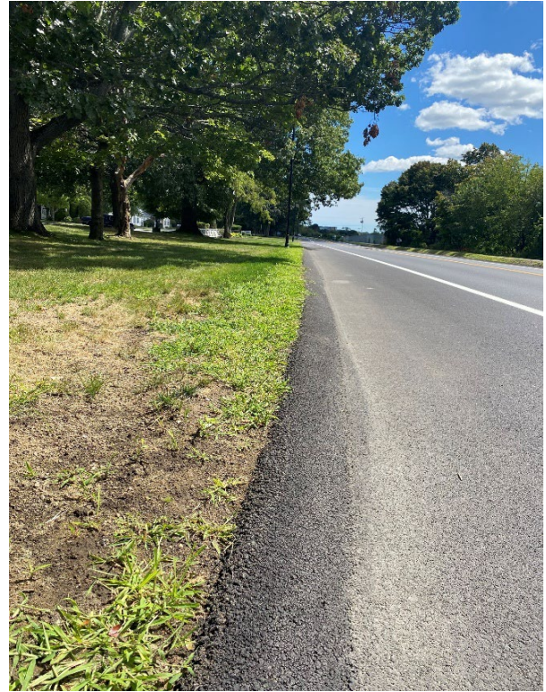
Figure 3-23 Appropriate for stormwater management. Berm along Veterans Memorial Parkway. Source: Pam Sherrill
