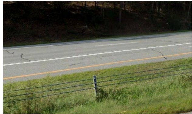
Figure 3-13. Steel cable guardrail along Route 1 in Charlestown, RI. Source: Elena Pascarella
